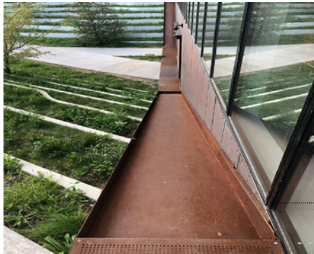
Gutter structure using similar materials as the exterior of the building near the entrance of bike parking
